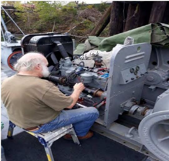
Steve installing wiring harness and water hoses onto newly rebuilt winch engine.
