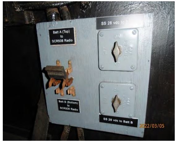
Restored Power Panel for Army Radios installed on the Conn. Restored by Mark and Jerry.
