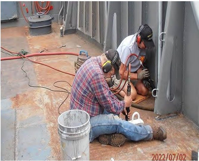
John and Sam busy chipping paint on Well Deck prepping for new paint.
