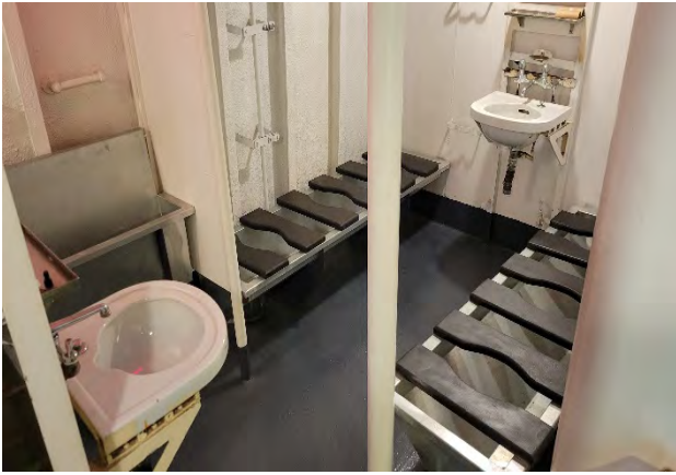
Crews Head - Toilet troughs and Urinal.
