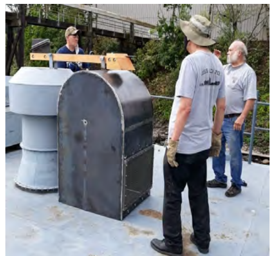
Ventilation duct, by Steve Adams (Affectionally "The Mailbox").
