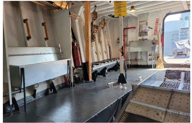
The Foc'sle- Troops: Urinal, Toilet Trough, Wash basin, (All, now operational).
