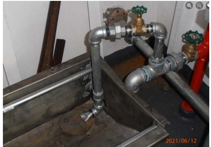
Flushing system for commode and urinal in ramp room for 'display only'.
