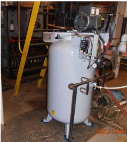
Heavier air compressor to drive the Master Blaster. Since nothing goes into the river, wiser paint removal methods are utilized.
