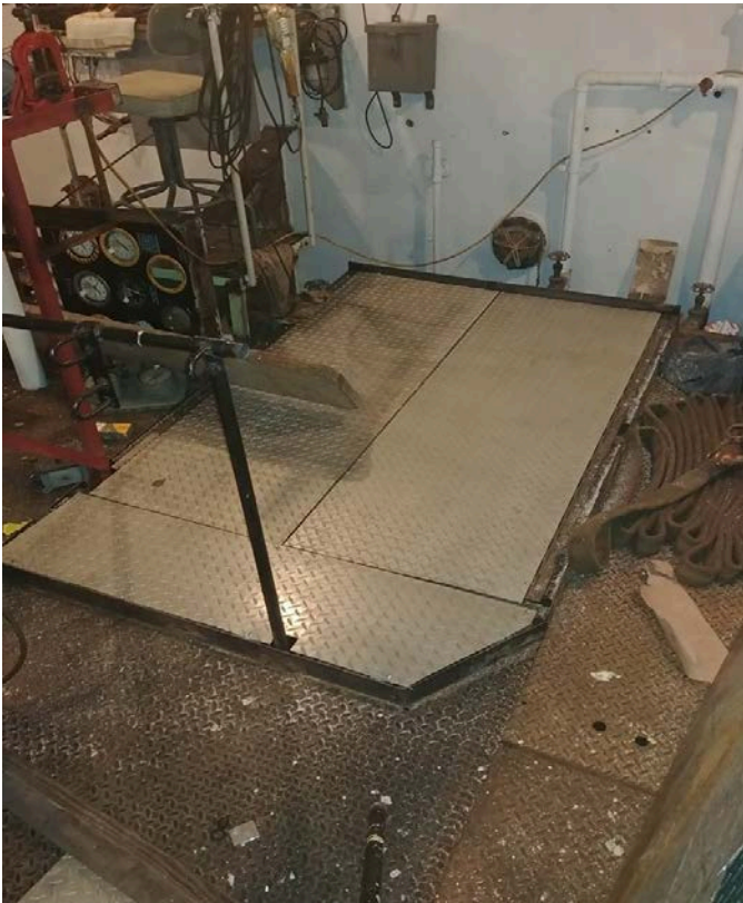
Engine room PORT side opening modified to fit 12V71 engine (in storage and ready). Hinged cover for safety. STBD is next.
