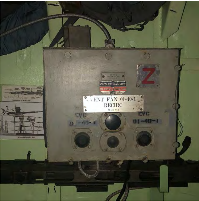
The fan control box in process of being connected in the original location in the Clipping Room beneath fan.
