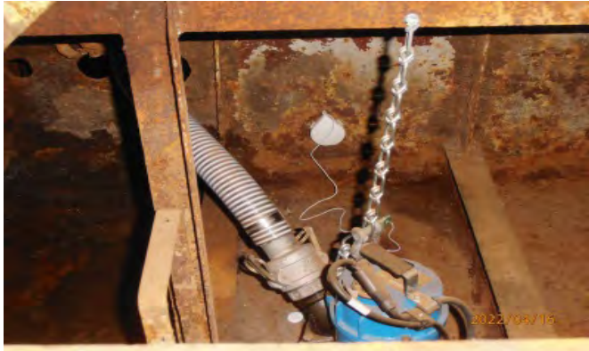
Here's what the pumps look like. The white circle on the hull bottom is the Moen water sensor.
