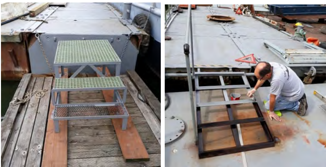
Repositioning of our Rhino barges and repair of our dock with additional floatation added.
