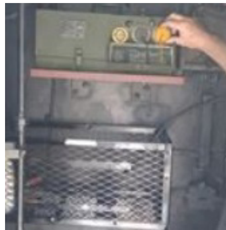
Battery powered bull horn racks were mounted inside the booby hatch.
