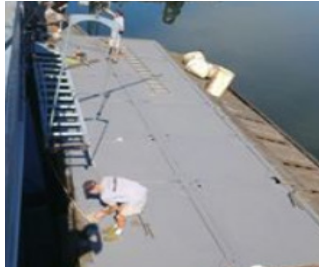
The wood floating pier has been re-floated and damaged portions removed. The second Rhino barge has been cleaned and painted and will be used as a secondary access to the LCI.
