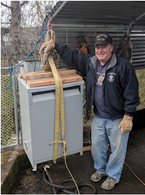
Jerry Gilmartin with our new transformer.
